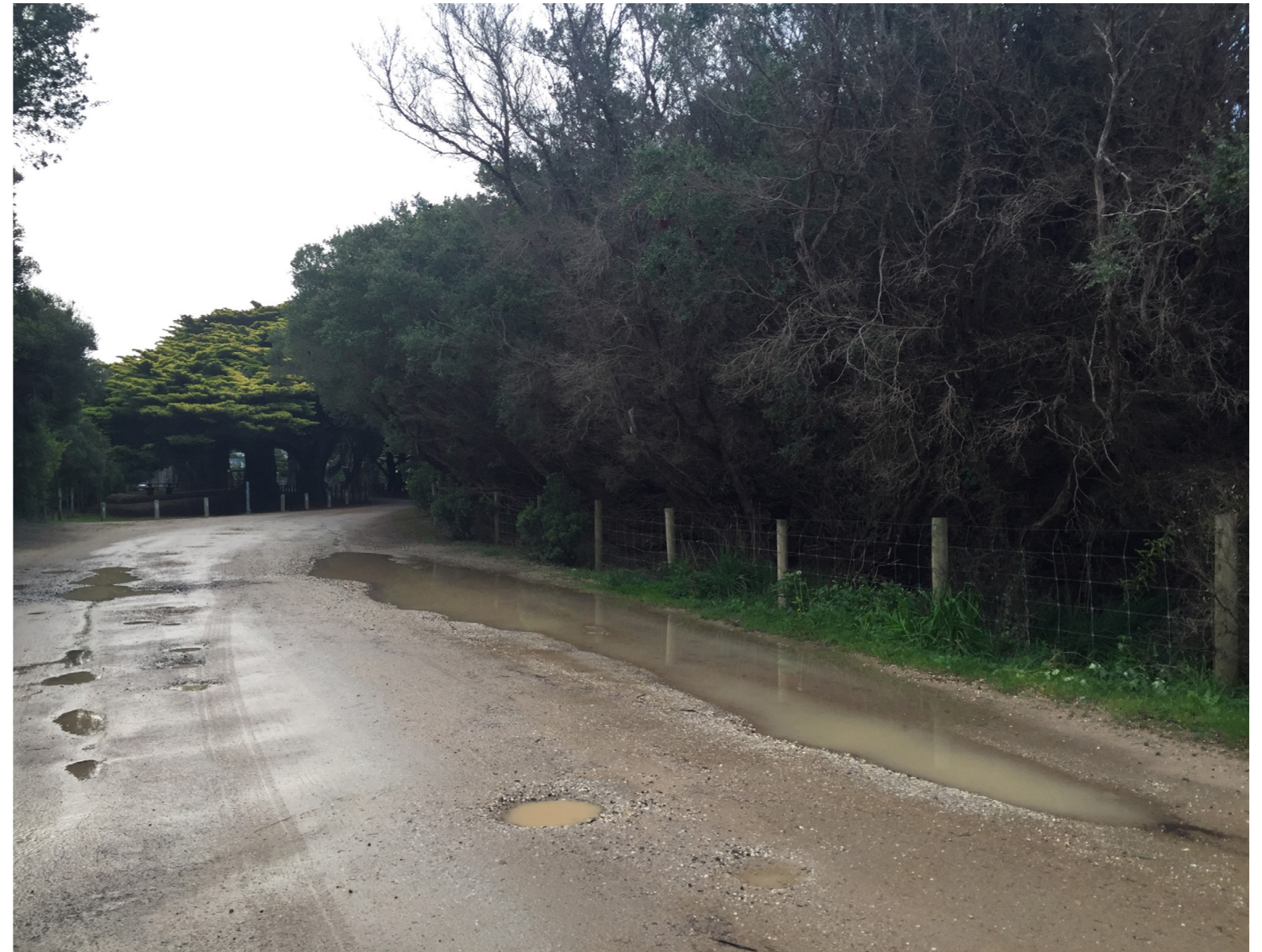
Staged removal of tea tree species to central island planting. Removal of between 0.5m and 1.2m of planting to eastern edge (as shown to right of image above) to allow for realignment of road, carparking and pedestrian path.
