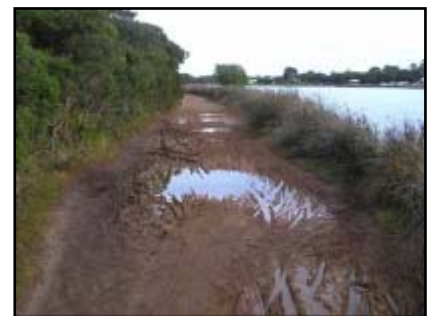
Severe track erosion in coastal heath (top), and near Anglesea River.
