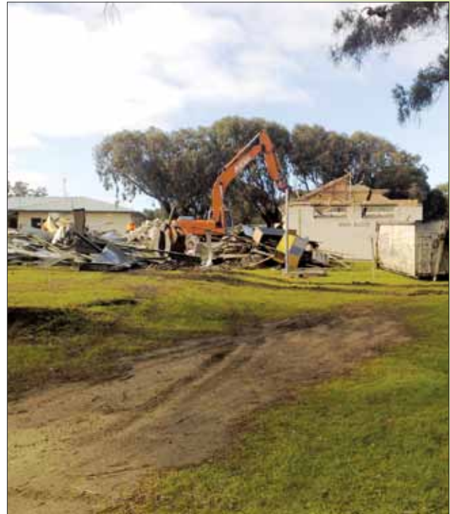
Torquay's ageing main amenity block was demolished in July 2009 to make way for a spacious new facility for campers.
